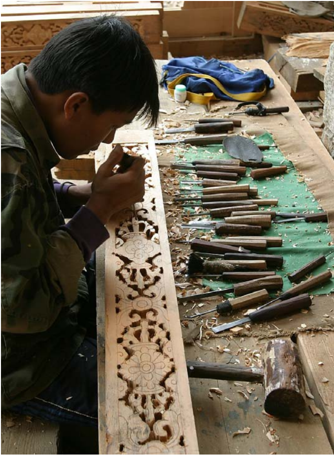
A master carver hand carving a beam for a new hotel being built in Paro, Bhutan. Note the hand formed wooden handled tools. Paro, Bhutan.
